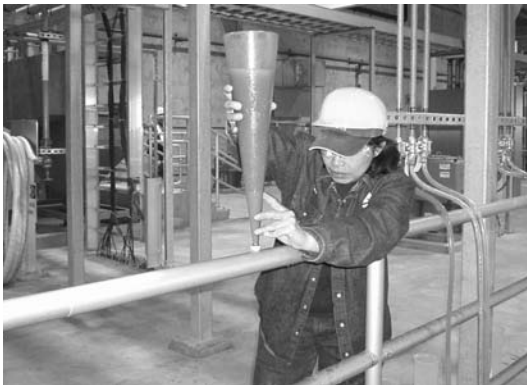
Surface water treatment plant operator checks the settling rate.
