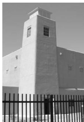
The raw water pump station.
